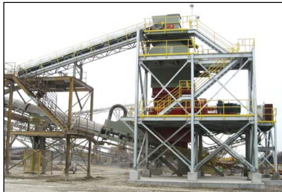
Part of new crushing and screening plant with dust controls being installed by Lafarge
